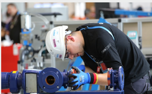
Pump maintenance and operation
